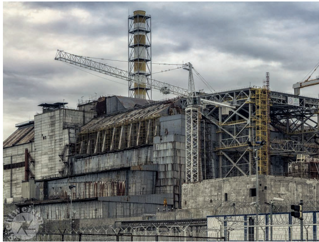
Figure 3. The “Cascade Wall” of the Sarcophagus in 2016 with the lost formwork from steel, now rusting, that was used to hold the concrete. Photo by Carina Buchspies (@sichtweisend).
