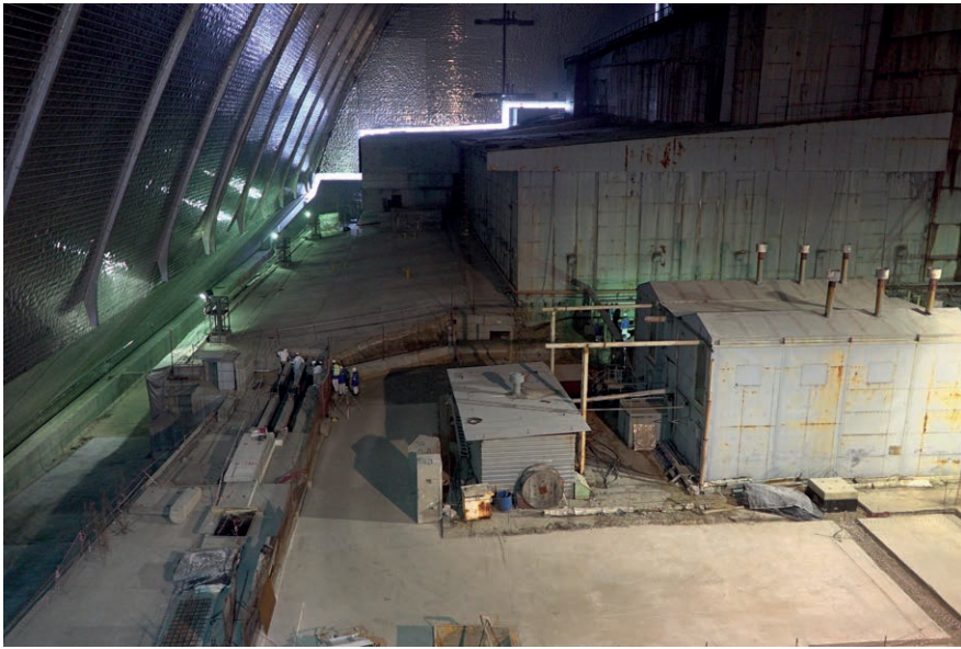
Figure 6. The preparation works (2016) within the New Safe Confinement before the sealing of the gaps between the old and the new structure. Courtesy European Bank for Reconstruction and Development (EBRD).
