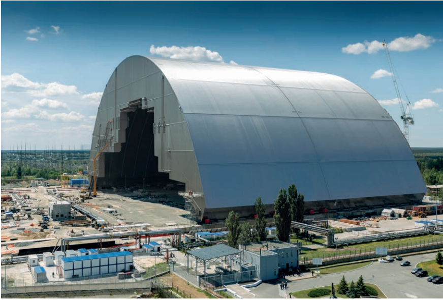
Figure 1. The New Safe Confinement steel structure in Chernobyl before being moved on top of the existing concrete Sarcophagus structure from 1986 that was poured onto reactor number 4. Photo by Francis Vigouroux, Courtesy Bouygues Construction.
