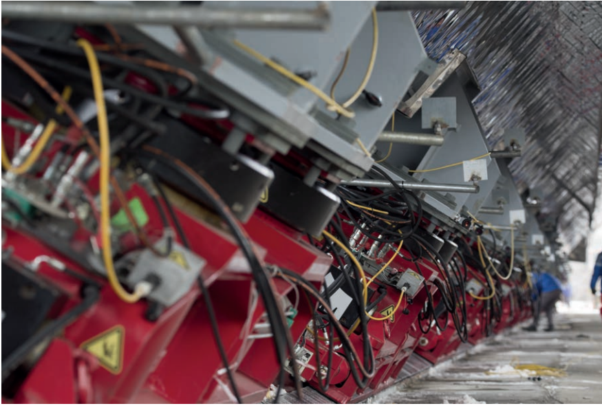
Figure 5. The synchronized jackhammers before the sliding operation in November 2016. Courtesy European Bank for Reconstruction and Development (EBRD).
