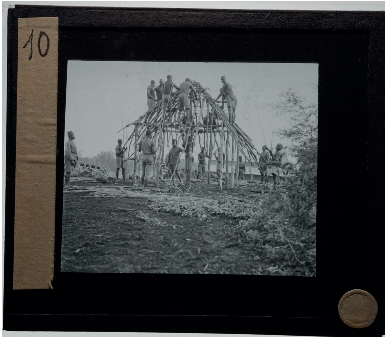
Figure 12. Construction of a meteorological observatory in Beni. "The observatory is built in matt. This type of house costs just a few francs."
